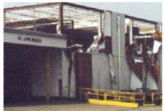
Old Lewis Bear Facility without Cornell doors - sustains heavy damage
