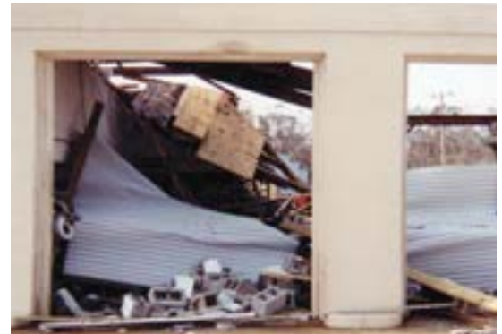
Severe building damage caused by substandard doors
