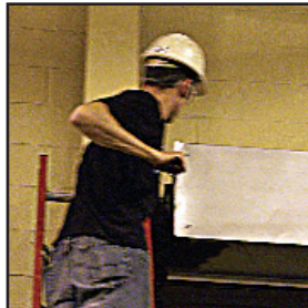
Installation of M100 Retrofit unit. Spring tension of door is temporarily relaxed.
