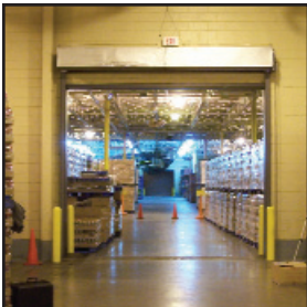
Typical conventional fire door mounted in a critical pathway. Downtime is costly and resetting is problematic.
