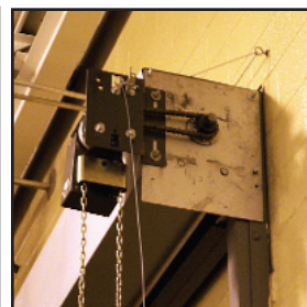
M100 Chain Operator installed and emergency ready.
