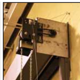
M100 Chain Operator installed and emergency ready.
